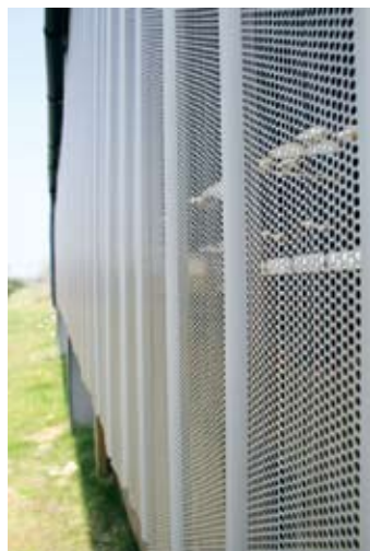
Perforated metal sheeting has improved air flow, while protecting against the elements at Pantswllt Farm.
